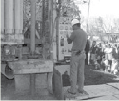
Crews broke ground on the new geothermal energy system at Parkway Terrace in November.
