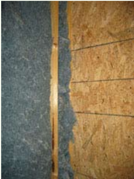
Insulation consists of a combination of closed-cell foam and cotton batting from recycled blue jeans.
